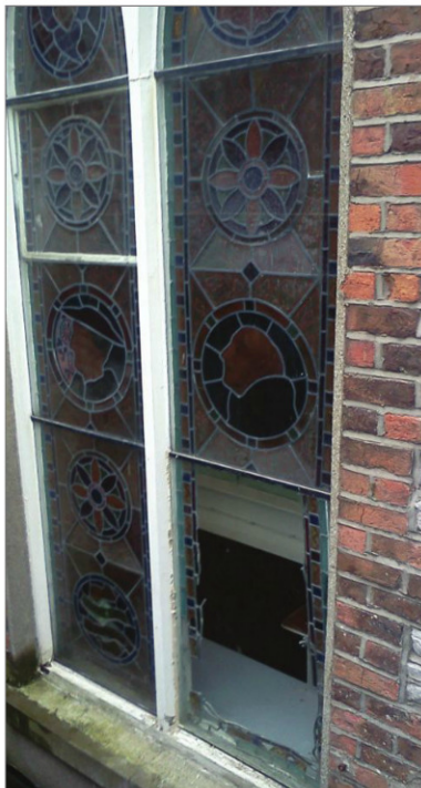
■ The window that was damaged.
